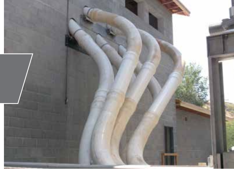
Six custom 12-inch pipes connect to a table on the second floor of the sorting room and snake their way to each raceway in the holding facility. A creative solution achieved by the Oxbow team, their supplier, and the design engineers. Soon fish will be making their way down the pipes as they are sorted to each raceway.
